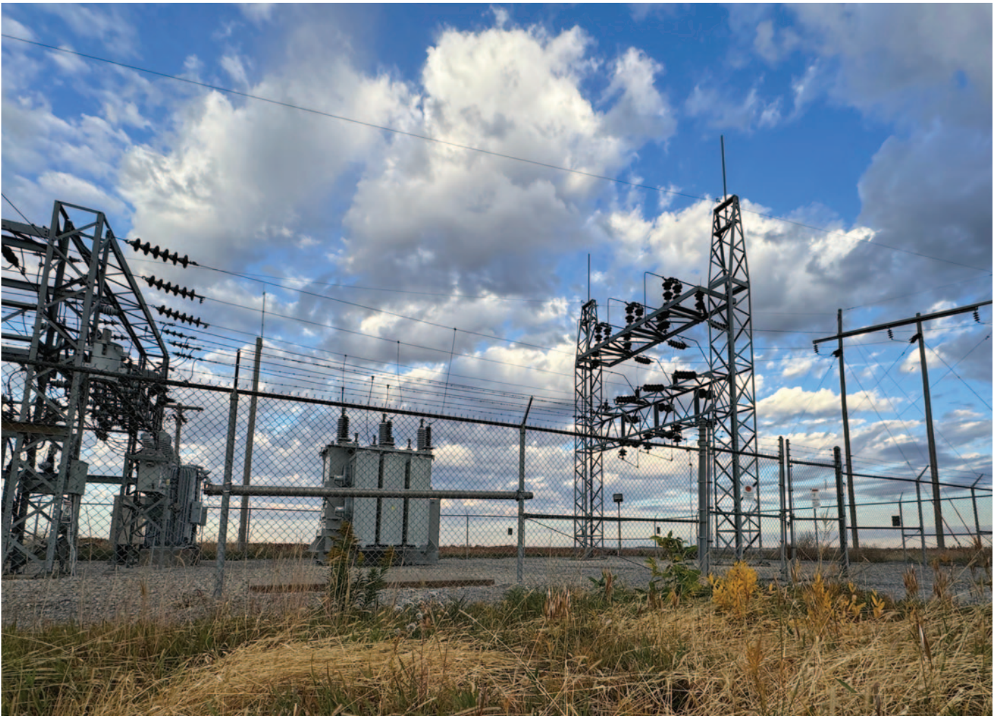
Substations serve as the quiet backbone of the electric system. Photograph by Barb Fowler, Polk County Rural Public Power District
