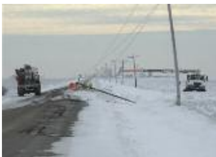
Strong winter winds can cause ice to build up on one side of a power line, causing them to bounce.
