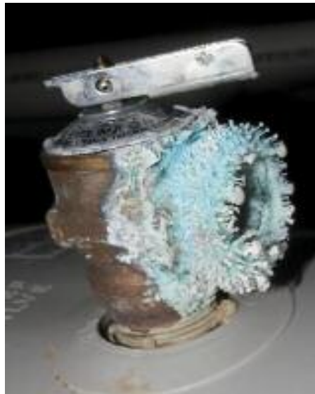
Mineral deposits on pressure release valves or corrosion on fittings coming out of the water heater are signs of leakage that should be addressed. Photograph by Jim Troth
